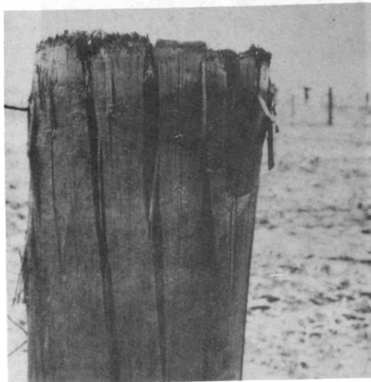
b. DAMAGE TO BUTT OF TIMBER PILE DUE TO HARD DRIVING
